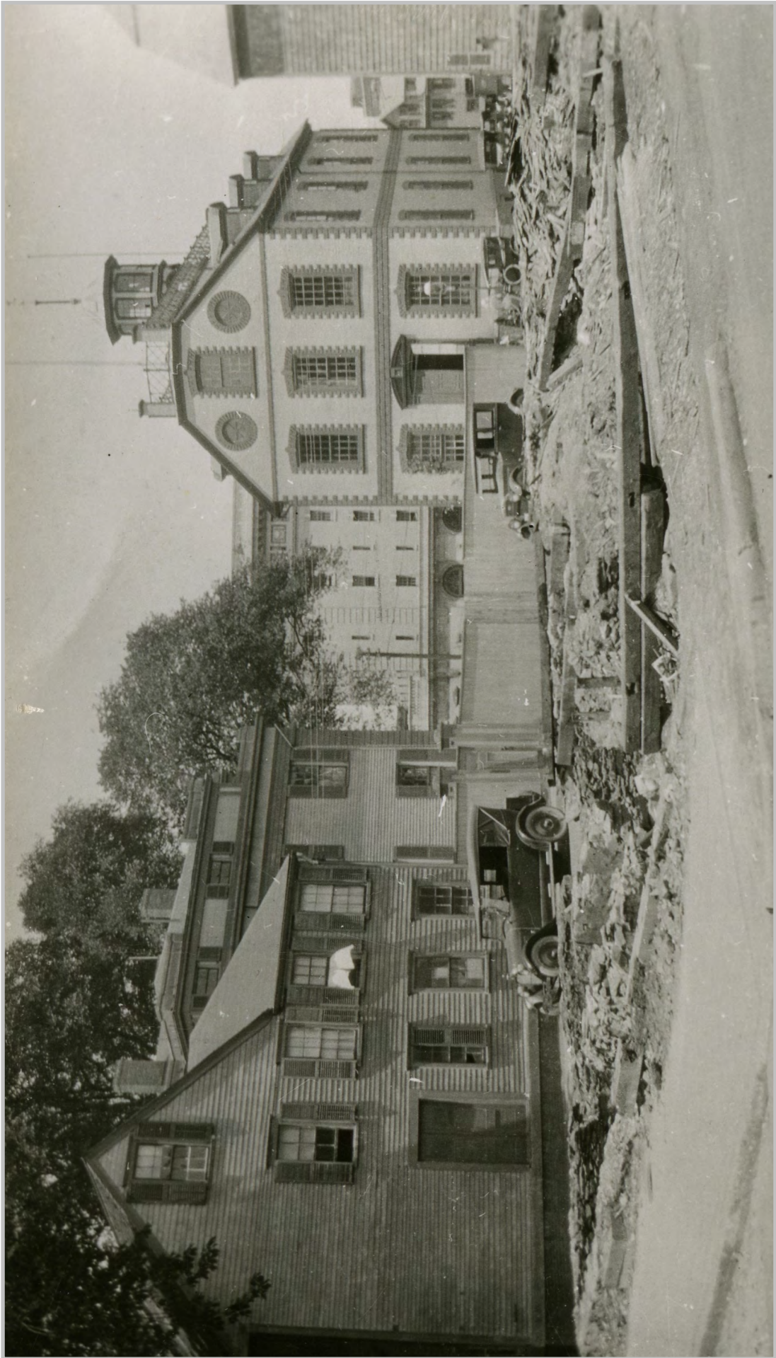
Demolition on the southern end of the future gas station site. Bliss House is located at left; Levi Gale House is to its right. Park House hotel has been demolished as well.
