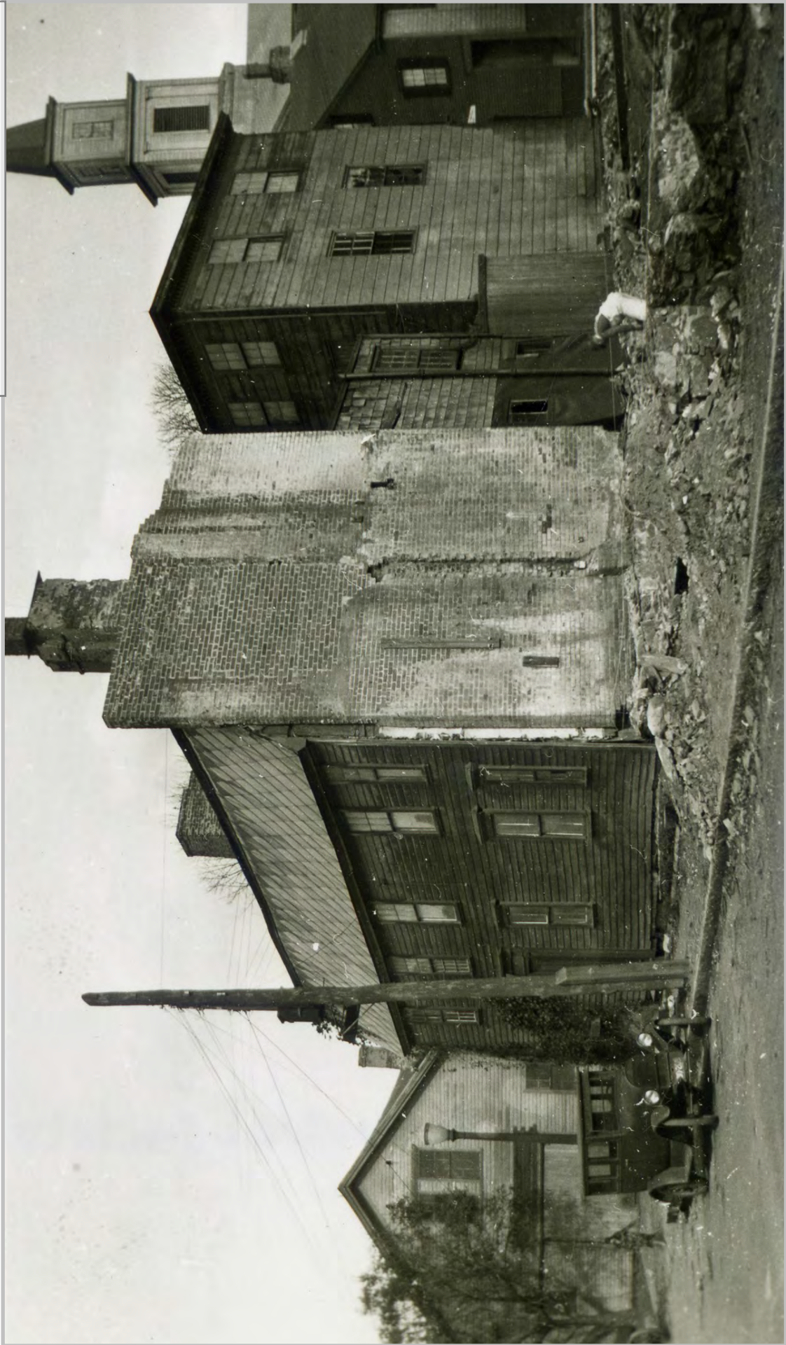
Demolition on the northern end of the future gas station site, looking towards Hozier Street.
